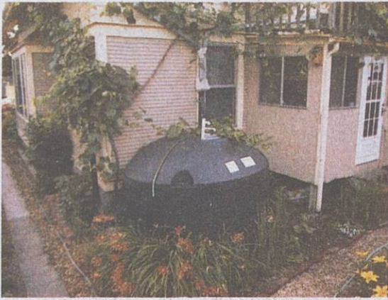
Rain water storage tank
